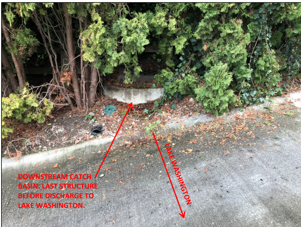
Figure III-7 – Trench drain near bottom of Holly Ln in front of 10 Holly Ln.
